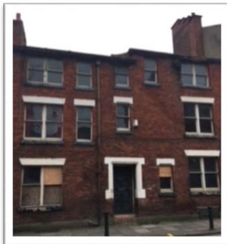
Figure 31: 6 Chapel Street, vacant and in a state of disrepair
