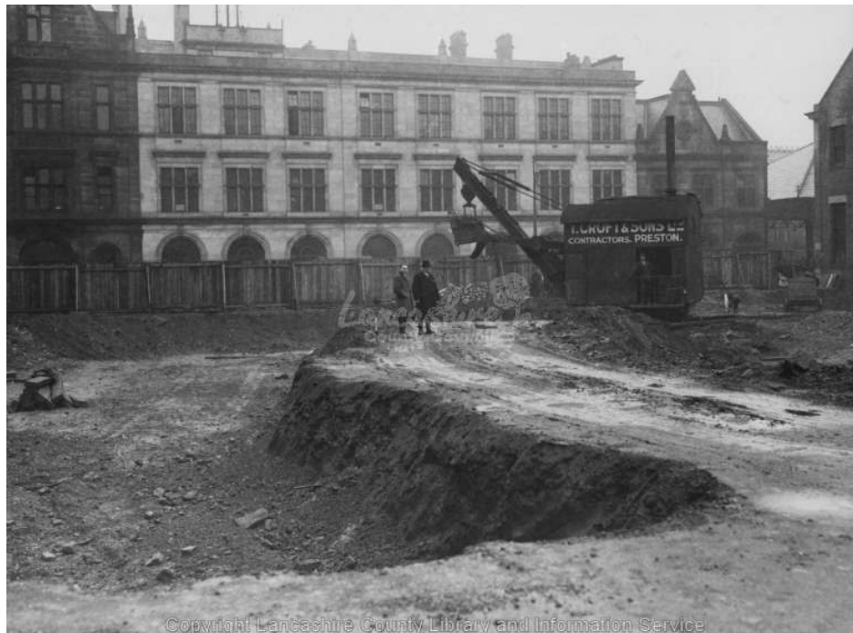
Fig 17 Photo c. 1931 showing the excavations for the Municipal Buildings, note the Post Office in the background
