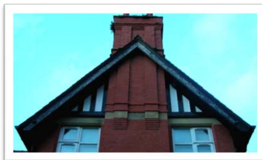
Figure 21 peeling paint on the timber bargeboards
