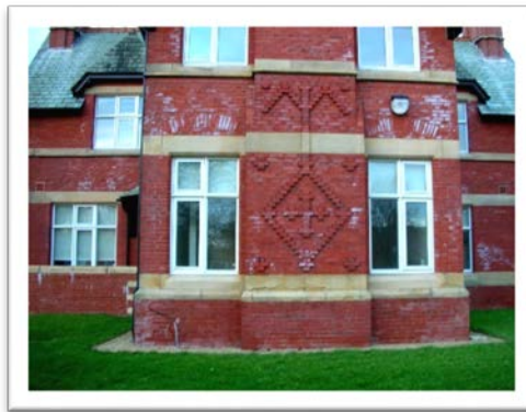
Figure 20 staining and efflorescence on the brickwork
