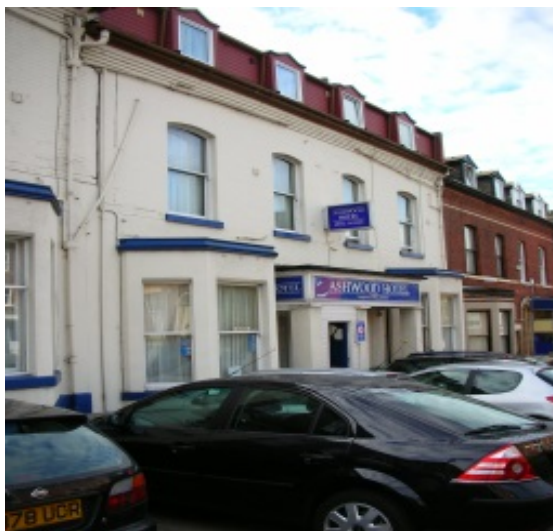
Exterior masonry paint can harm the appearance of a uniformed terraced
