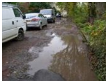
Private Road in Poor Condition
