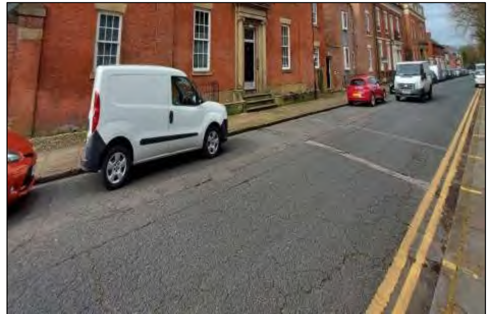
Unmaintained street surface with evidence of repairs (West Cliff).
