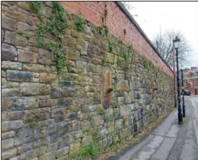
Brick and stone boundary treatments located on West Cliff terrace, associated with the Railway
