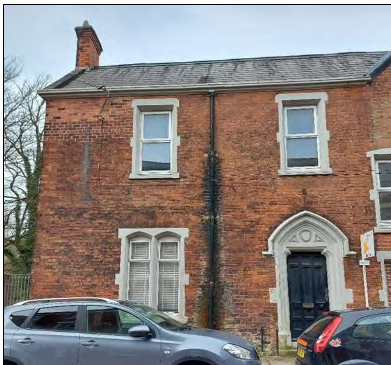
Damaged rainwater goods
