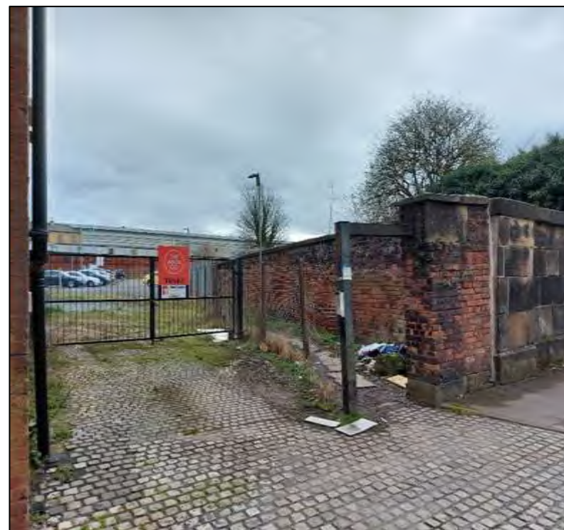
Lack of maintenance of a car park and alleyway
