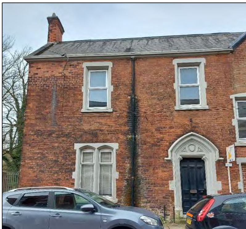
Damaged rainwater goods
