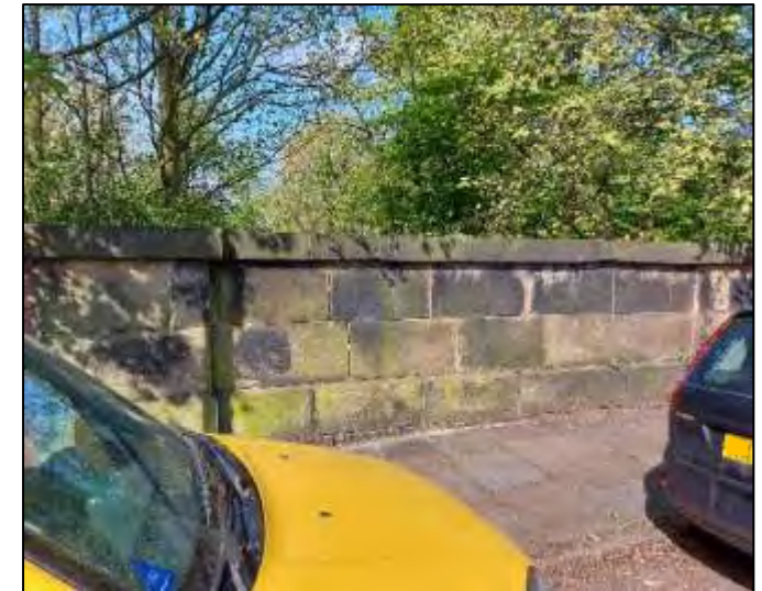
Stone treatments to the bridges that traverse the disused Ribble branch railway
