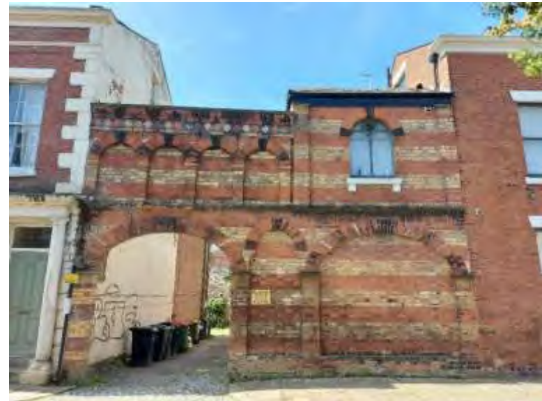
Polychrome brick wall on Latham Street and plastered quoins at either end of 22-28 Latham Street
