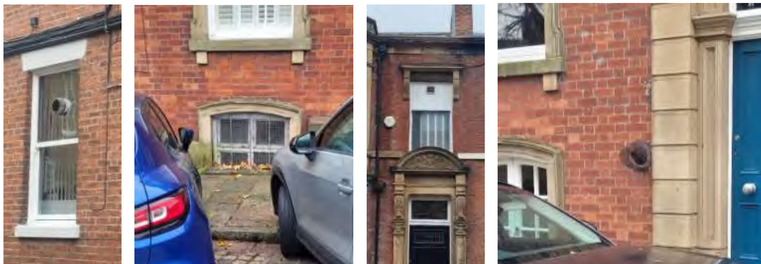
Vent in a window at Camden Place (left), security screen on window at Avenham Colonnade (centre left), altered window with vent at Ribblesdale Place (centre right), vent in wall at 5 Avenham Colonnade (right)
