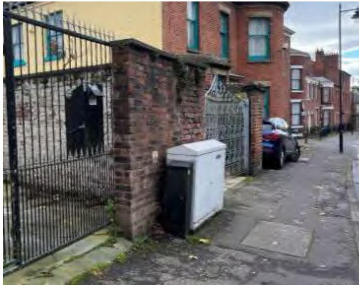
Utility box along Avenham Lane
