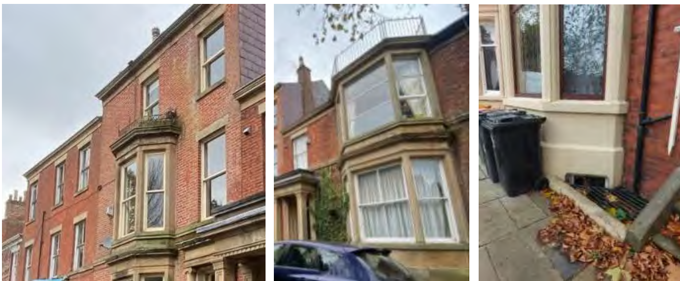
4 Bank Parade railings above canted bay window (left), 3 Bank Parade railings on the roof (centre), iron gratings covering basement level at Bairstow Street (right)
