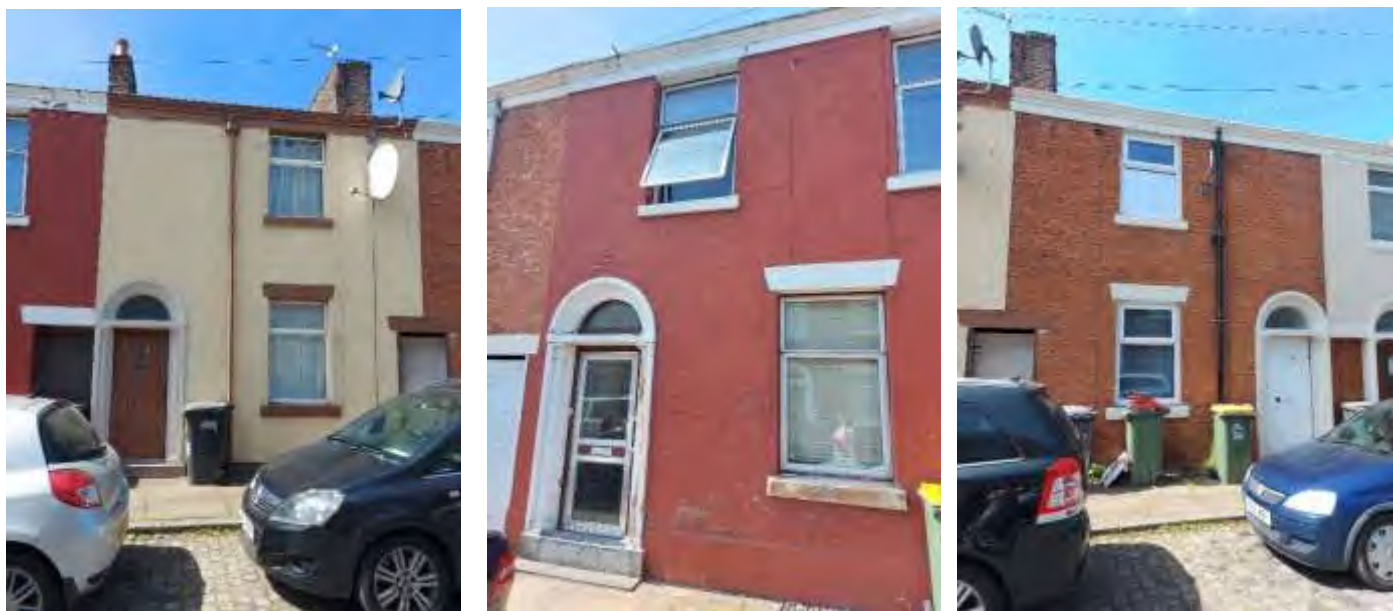
Incompatible door and window alterations, use of metal and uPVC along Frenchwood Street
