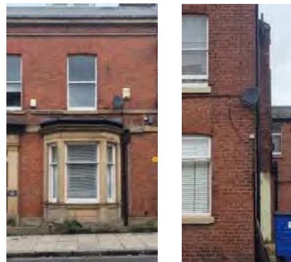
Satellite dishes and cables
