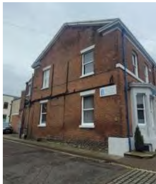
Brick discolouration (possible damp)
